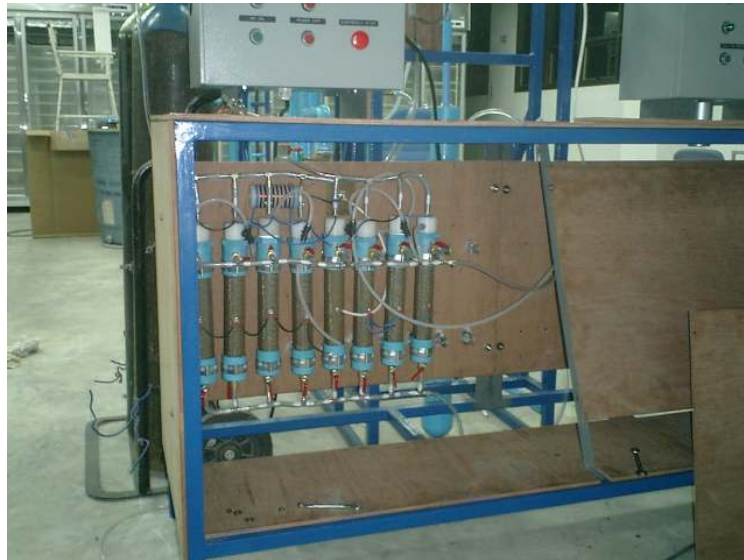
Figure 2 Eight ozoniser tubes connected in series to produce maximum ozone concentration.
